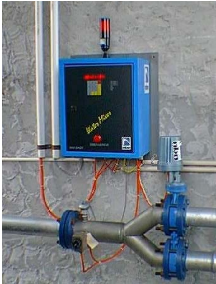
Figura 1: Base do Water Mixer instalada
